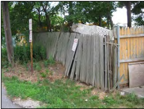
Photograph 9: View of deteriorated fencing along Garrity Avenue.
