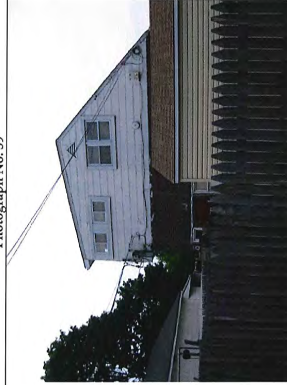
View of possible associated residential use, minor siding deterioration.
