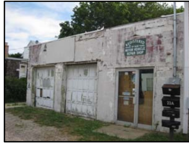
Photograph 1: View of deteriorated building along the east side of Hawkins Avenue.
